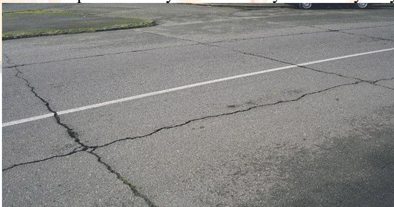
Fig. Joint Reflection Cracks
