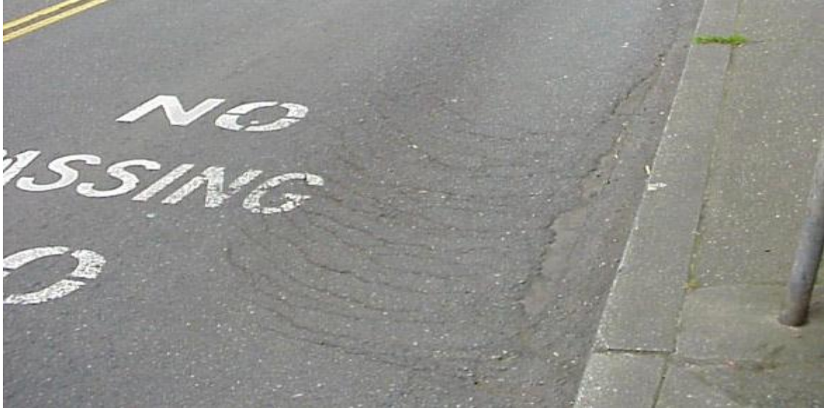
Fig. Slippage Cracks
