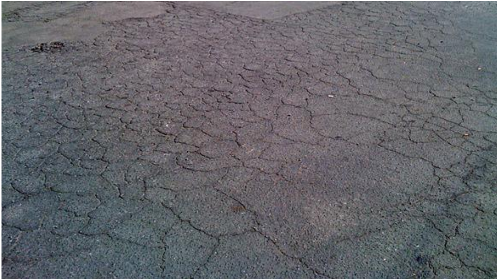
Fig. Alligator Cracking
