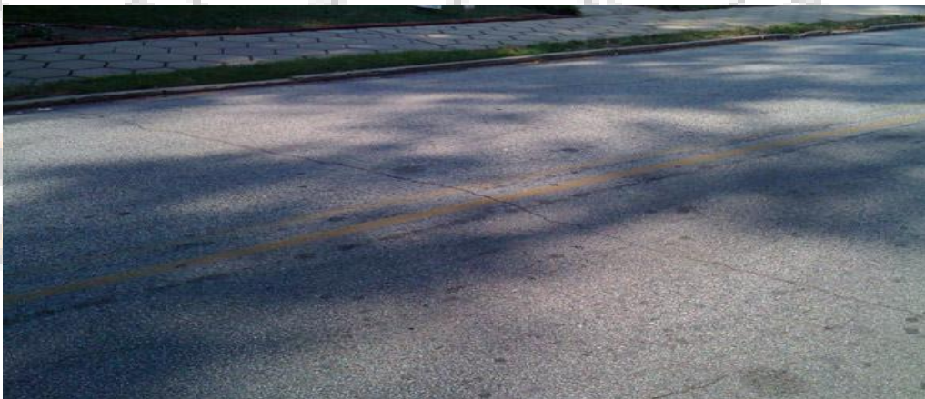
Fig. Transverse Cracking
