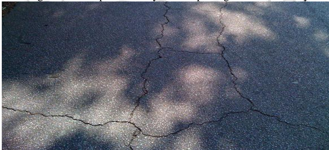
Fig. Block Cracking
