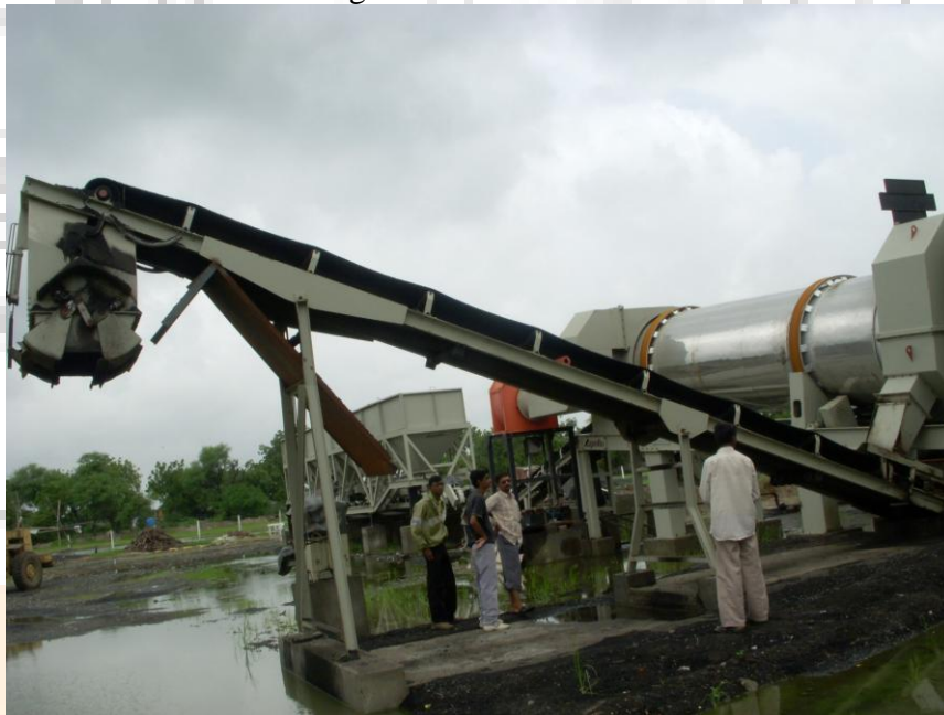
Fig. Load Out Conveyor
